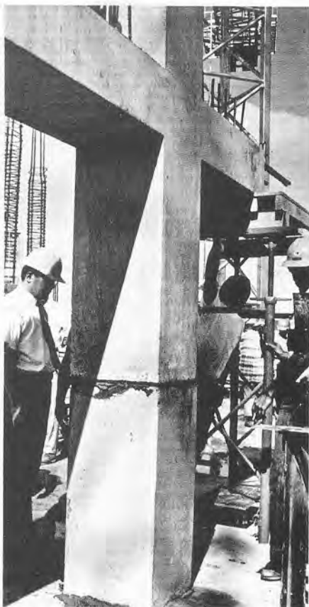
Fig. 3. Splicing H shaped precast units. The special high strength grout is visible around the joint between the two H frames.
