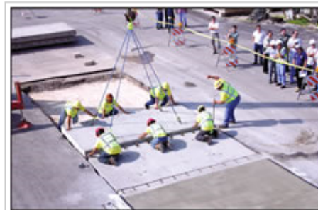
Photo from Grace Pacific A crew installs one of Yee's Kwik Slabs
